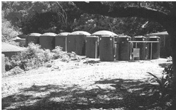
Modular Process Stream - Treatment Plant site
