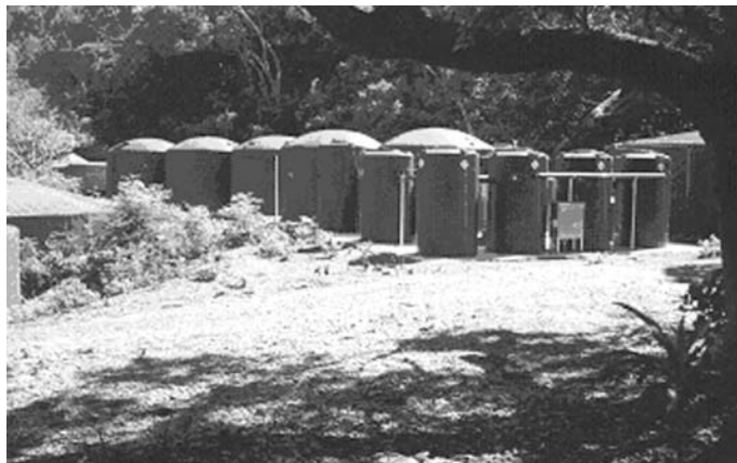
Modular Process Stream - Treatment Plant site
